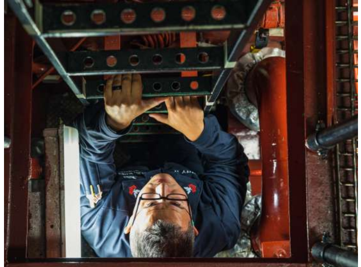
Machinist Mate 1st Class Richard Terry II climbs up a ladder in the main engine room of USS Paul Ignatius (DDG 117), Aug. 5, 2022. (Photo by Mass Communication Specialist 2nd Class Aaron Lau)
