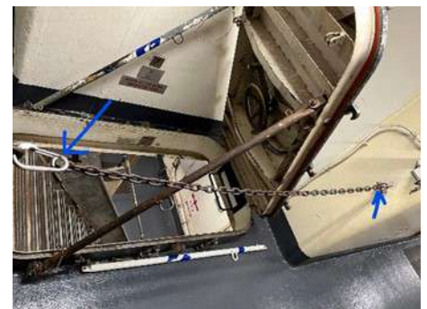
Above, left: Additional examples of improper installation, maintenance and construction of lifeline chains.
