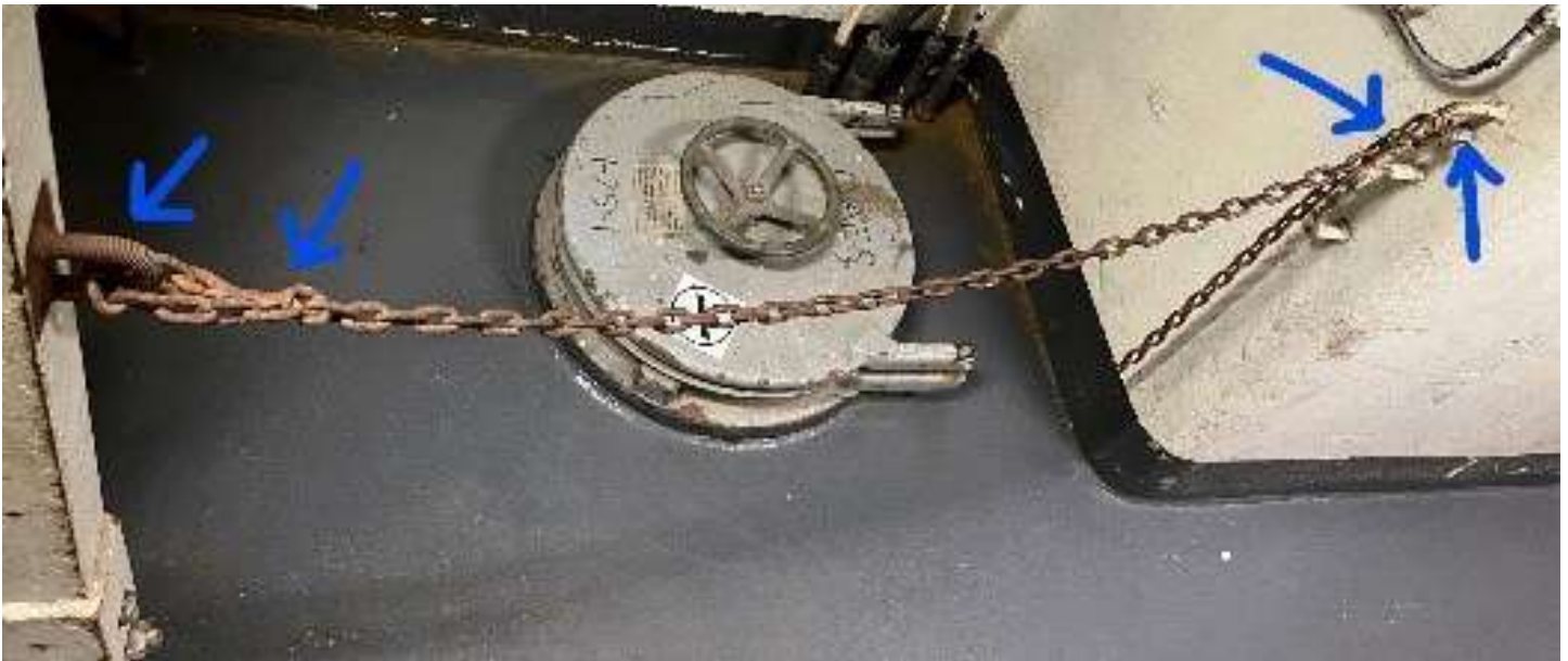
An example of improper installation, maintenance and construction of lifeline chains.
