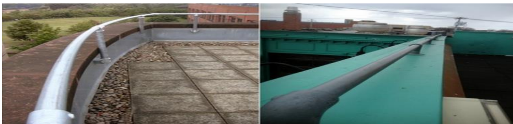
Above, solutions using additional railing to make parapets comply with OSHA 42-inch height requirement.
