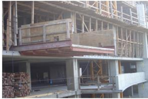
Loading Platform w/Removable Chain at point of access, however Mid Rail is also Required
